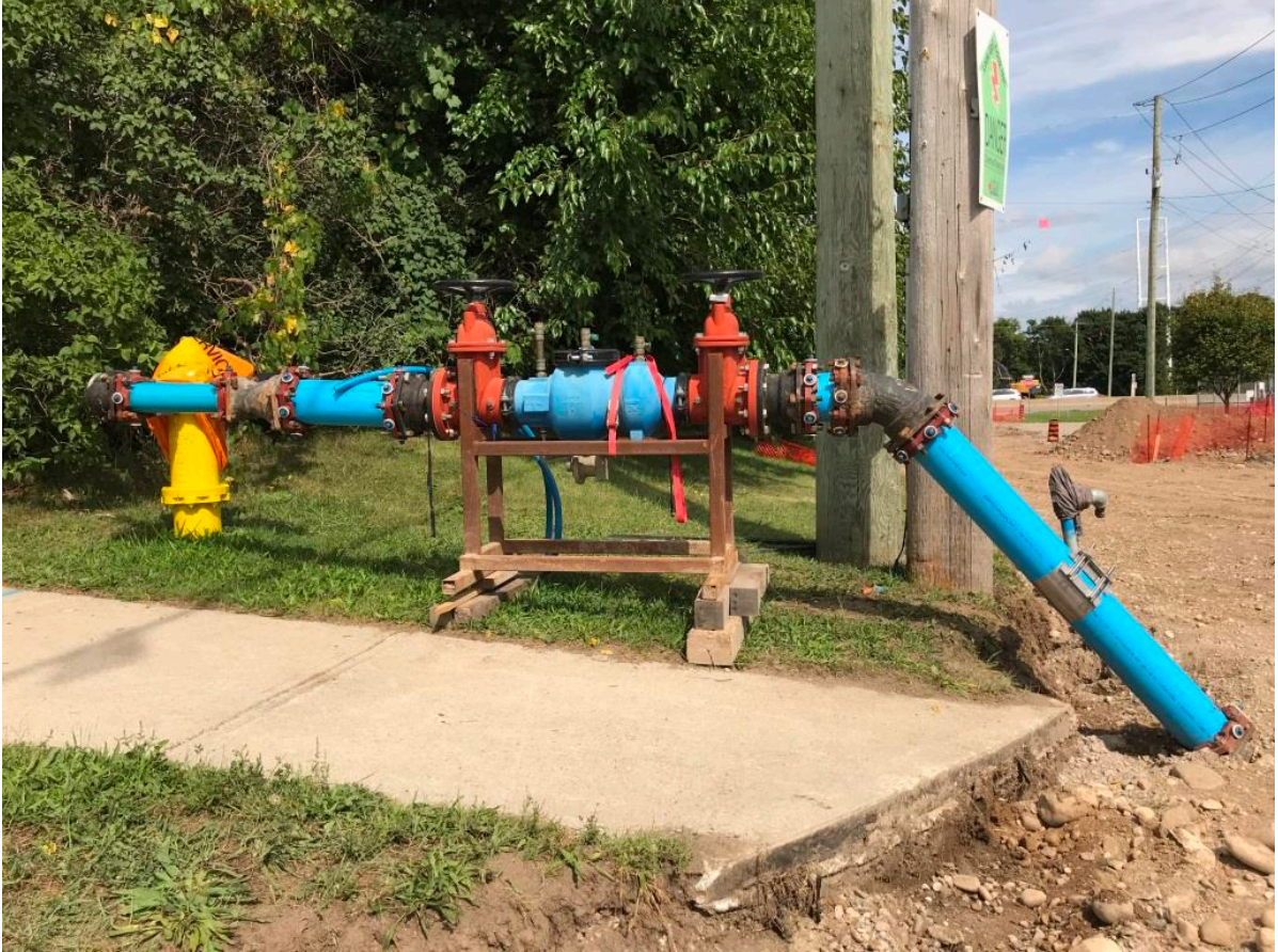
Figure A-1: Temporary connection from a hydrant with Backflow Prevention using a CSA-certified reduced pressure principle backflow preventer.
