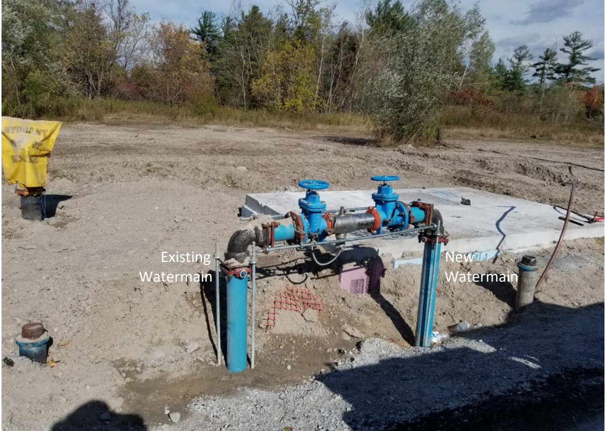
Figure A-2: Temporary connection from a watermain with Backflow Prevention using a CSA-certified reduced pressure principle backflow preventer.
