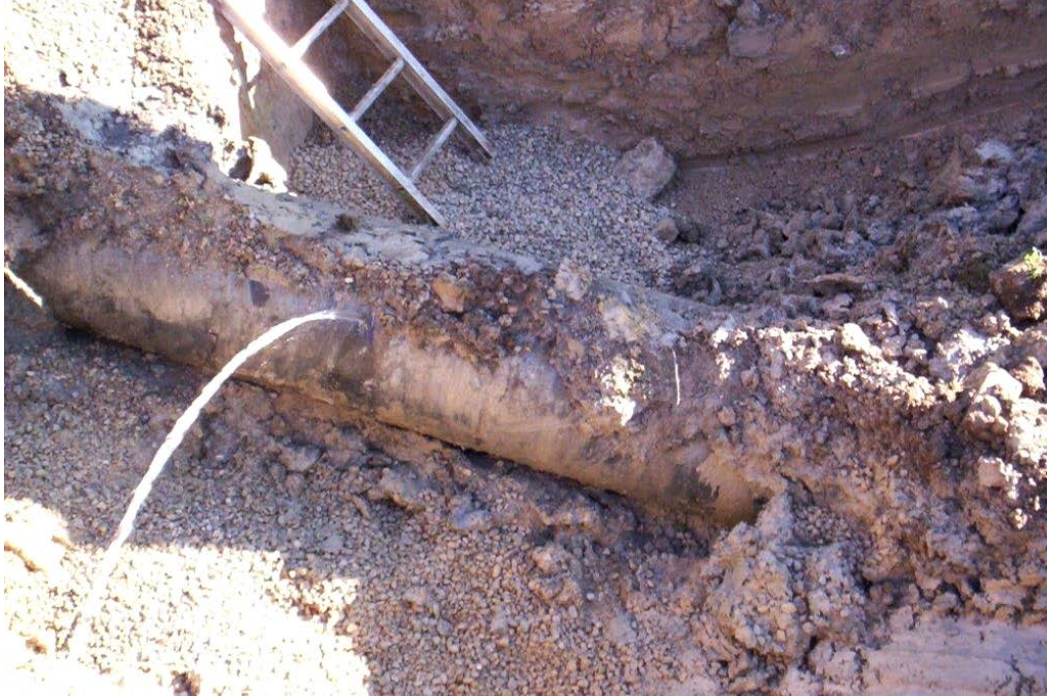
Figure D-2: Corrosion hole leak in a watermain with flow maintained until after an Air Gap was established.
