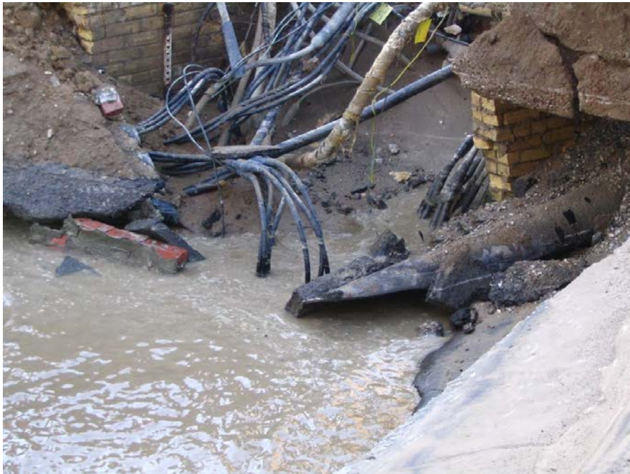
Figure D-4: Spiral watermain break with evident Contamination.
