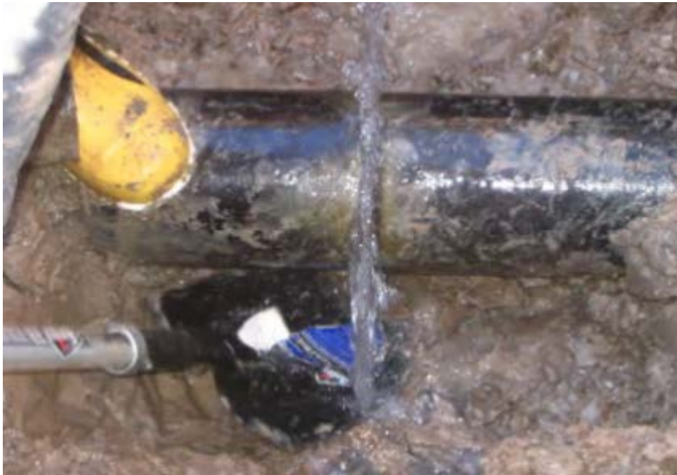
Figure D-1: Circumferential watermain break with flow maintained until after an Air Gap was established.
