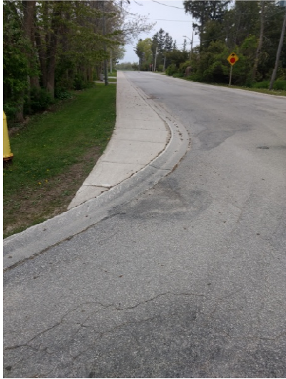
Trip 77 - Along Entry Curb Potentially
