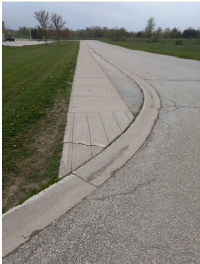
Trip 79 - Along Entry Curb Potentially
